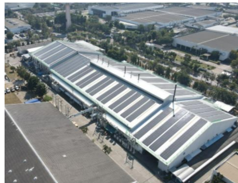
Solar power generation facilities installed at the Thailand plant
