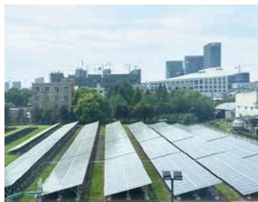
Solar power generation equipment installed at a manufacturing factory in China
