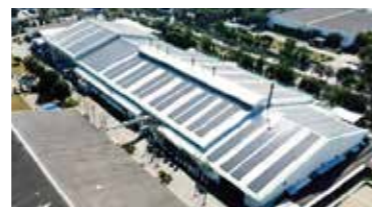
Solar panels installed at a factory in Thailand (ECT)
