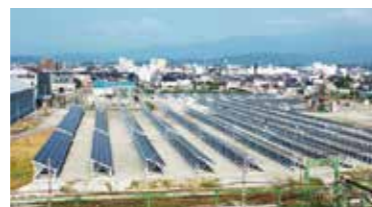
Solar panels installed at Uozu Factory
