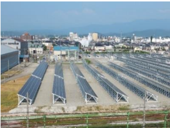
Solar panels installed at Uozu Plant
